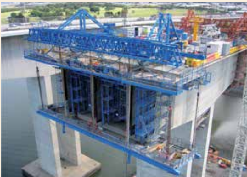
The form-traveller design provided excellent access to all the required working areas and allowed placing of prefabricated web reinforcement.
