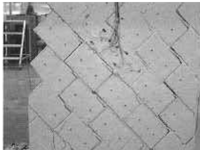
b) Sliding failure along joints
