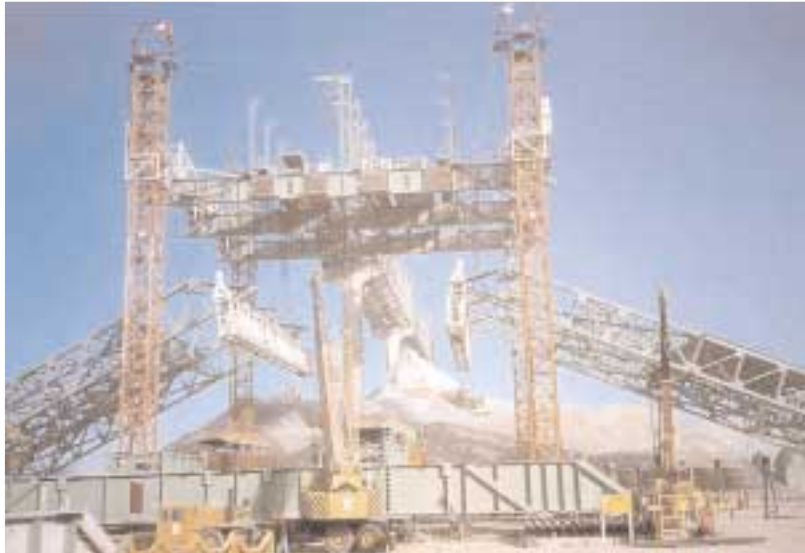
20,000-m 2 steel roof structure, weighing 4,200 t. For erection using the lifting method, the steel roof structure was divided into 8 sections.
