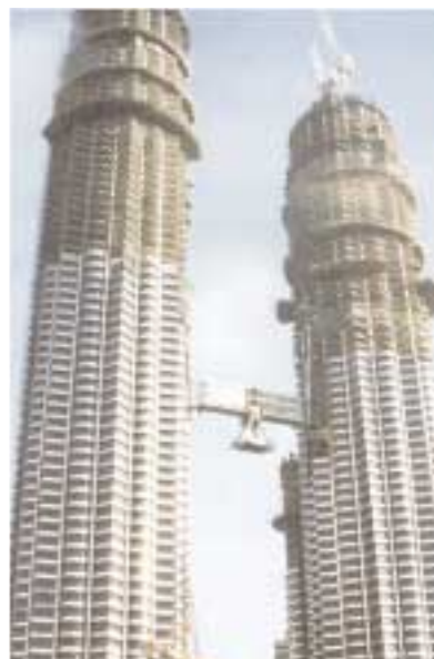
Lifting of the skybridge to link the two Petronas Towers on level 170 m
