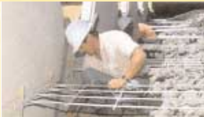
4 • Connecting the mesh with the loop clevis thanks to a dowel bar
