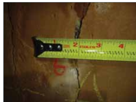
During an internal visual inspection in 2013, Tucson Water crews identified a pipeline leak as water penetrating into the 84-in. PCCP wall from the outside. Photo courtesy of Hector Posada, Tucson Water.
