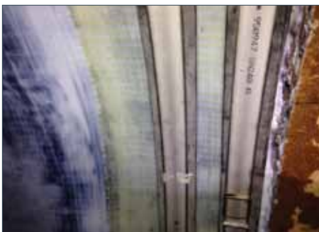
The best practice for end detailing of CFRP systems includes a specially designed leak-tight connection through a tie-in at the steel cylinder portion of the PCCP. Photo courtesy of Hector Posada, Tucson Water.
