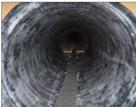
The CFRP installation was completed successfully and safely by Structural Preservation Systems, LLC, using CFRP materials supplied by Structural Technologies, LLC, both Structural Group companies. Photo courtesy of Hector Posada, Tucson Water.
