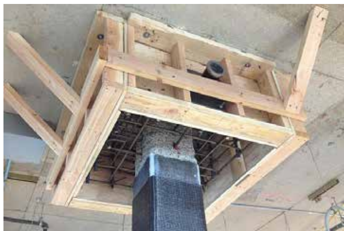
Columns wrapped with FRP for axial strength and enlarged for punching shear.
