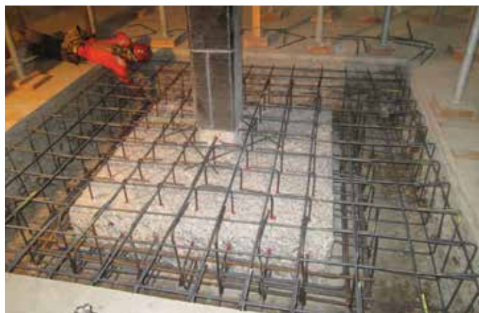
Enlargement systems were used to strengthen the column footers in the parking structure.
