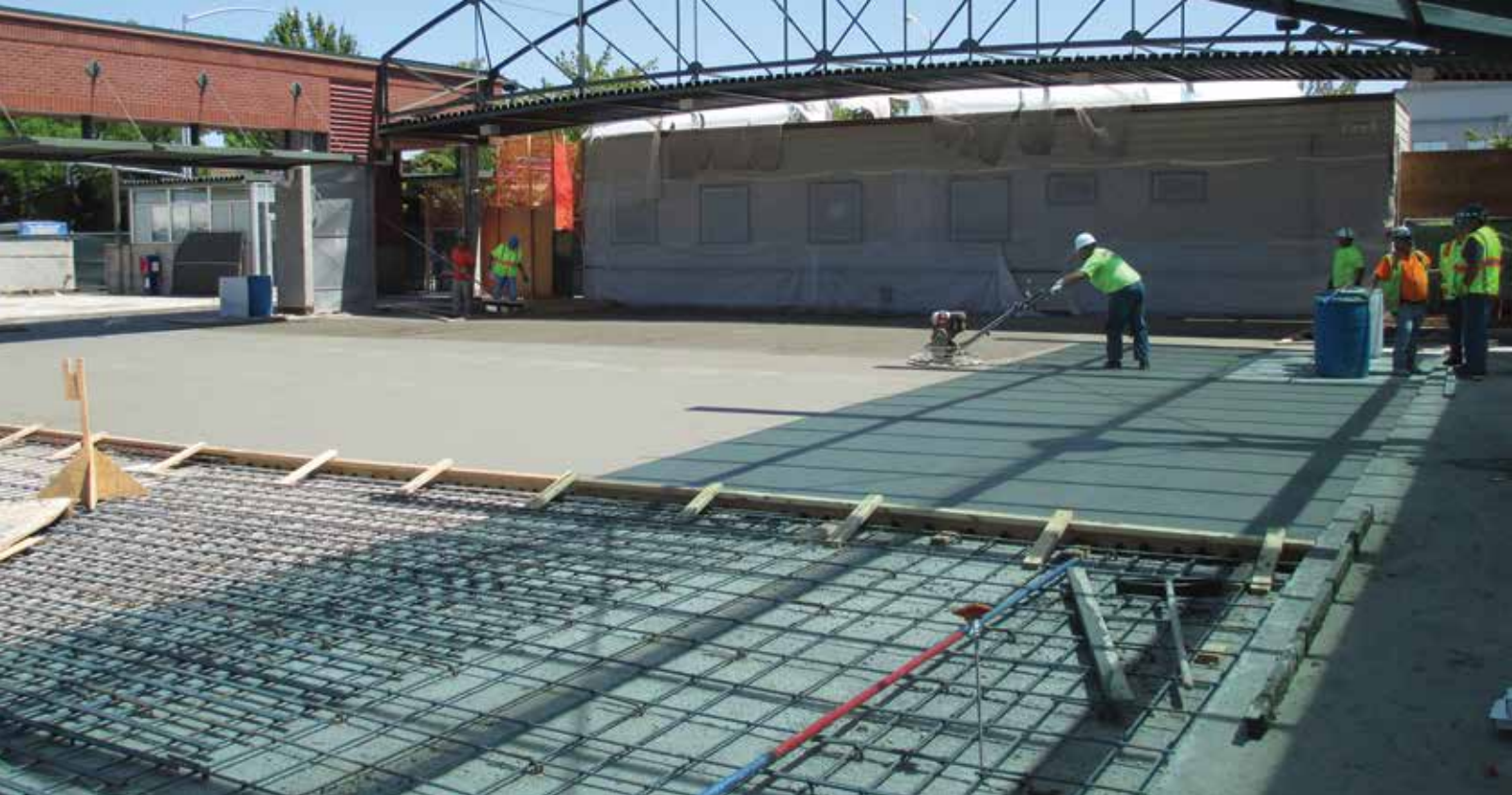
Placement of bonded overlay over the parking structure created a strengthened deck for the public transportation area.
