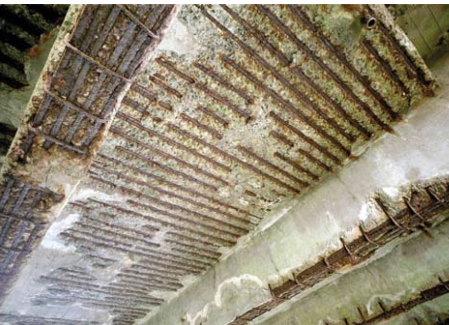
Corroded reinforcing steel in concrete deck
